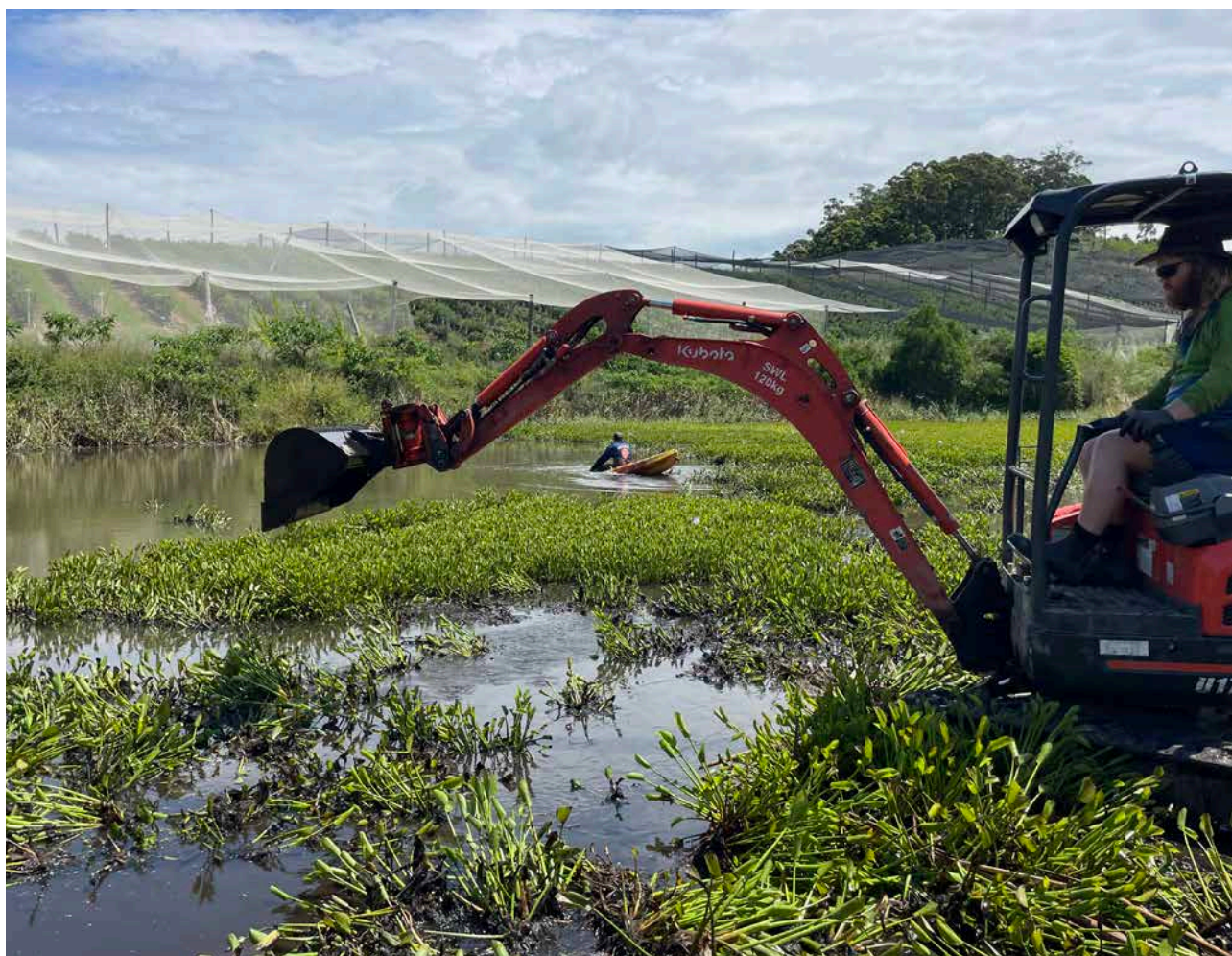
Figure 6. Mechanical removal of aquatic weeds using an excavator. Photo credit: Melinda Simpson, NSW DPI
