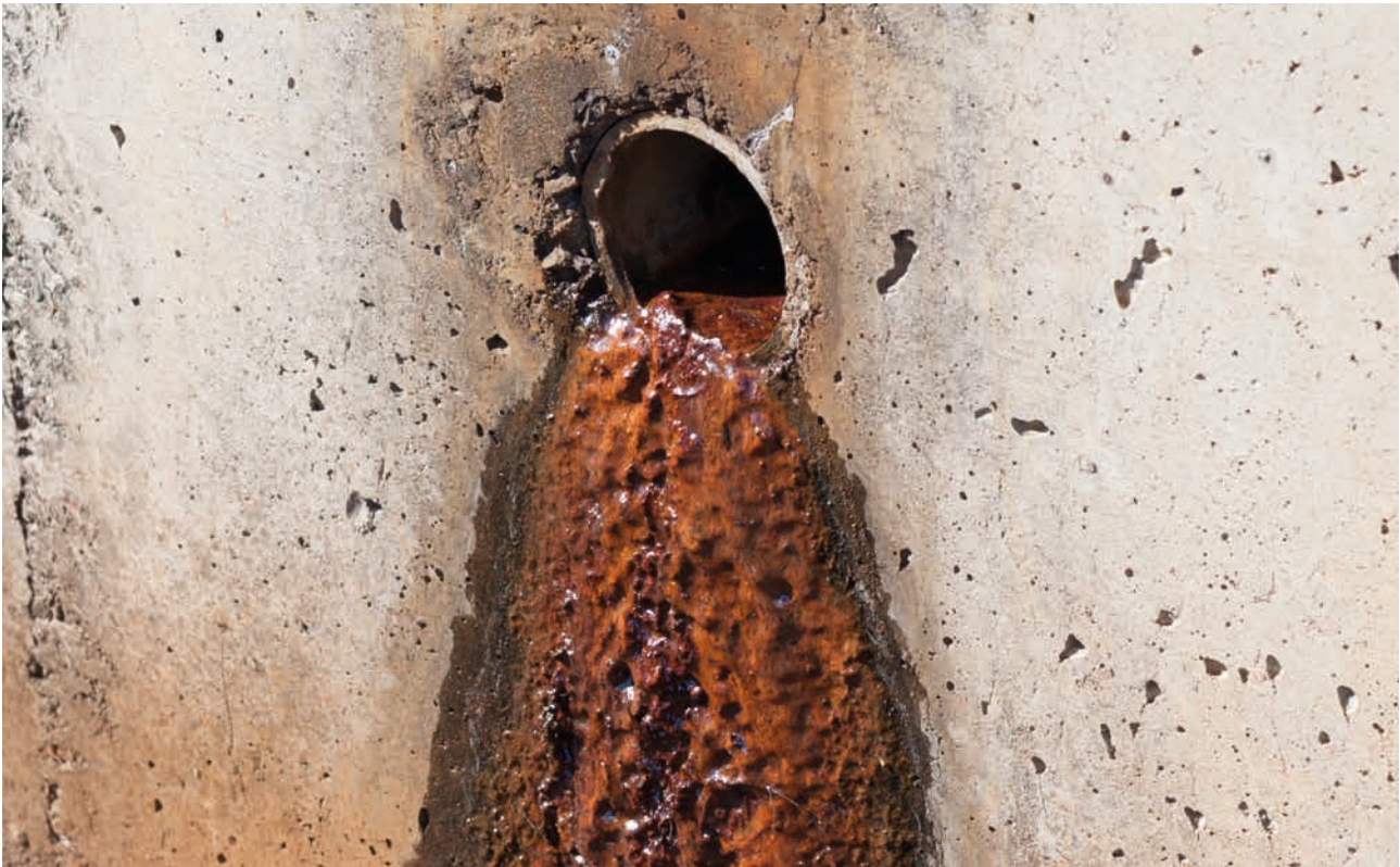
Figure 8. Iron sludge in pipe. Photo credit: Canva
