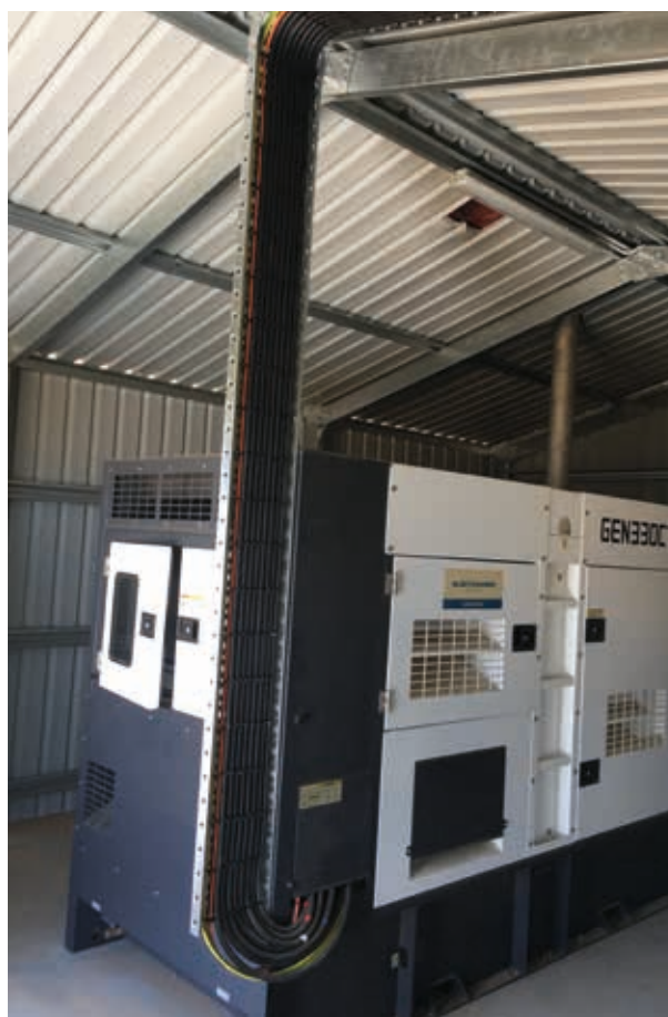
An example backup power generator installation that sits inside a dedicated shed space to keep it secure and protected from weather.
