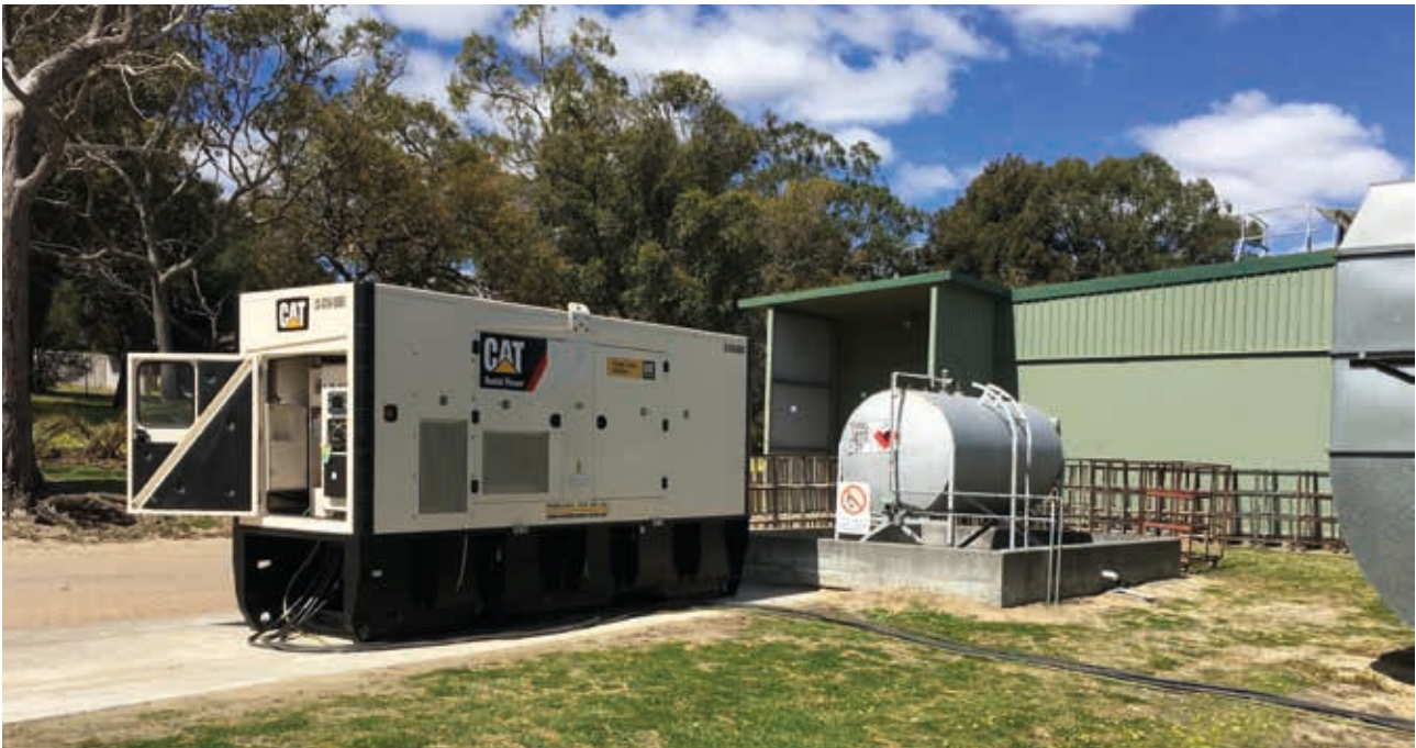
An example diesel backup power generator installation that can be sited outside. Photo credit: BON Electrics
