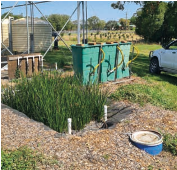
Figure 2. Reed bed in foreground and bioreactors in background
