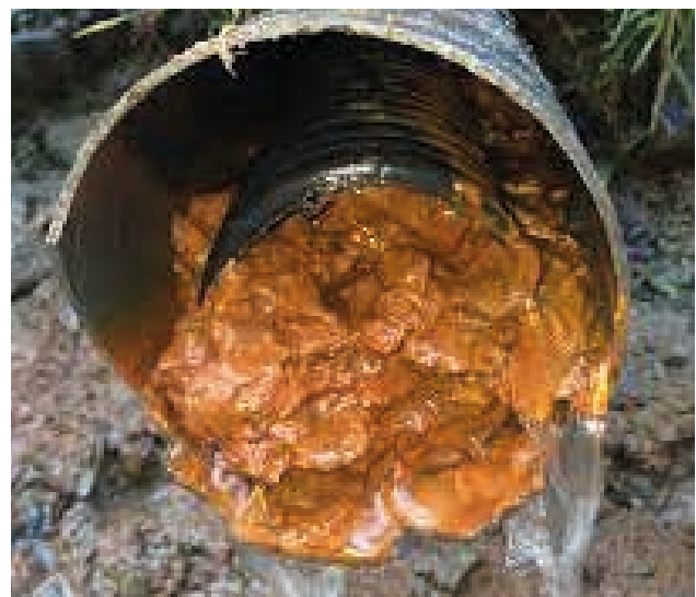
An extreme case of iron sludge deposits inside a pipe.
