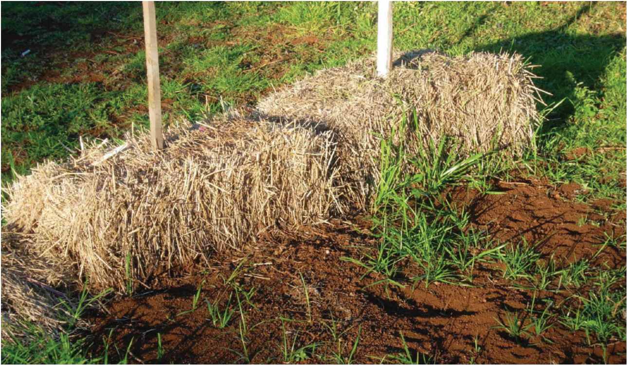
Figure 3. Hay bales placed as an erosion control method. Photo credit: NSW DPI
