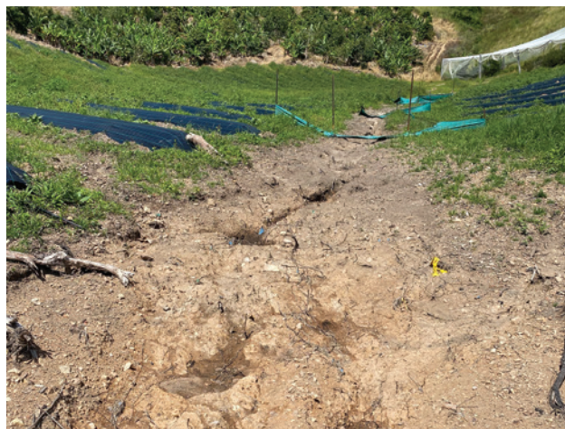
Figure 2. Erosion from large volumes of fast flowing water.
