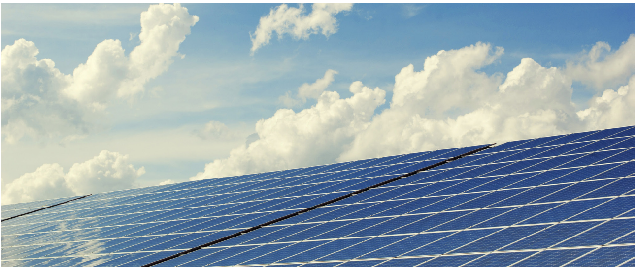
A solar installation can generate significant energy use savings. Photo credit: Pixabay
