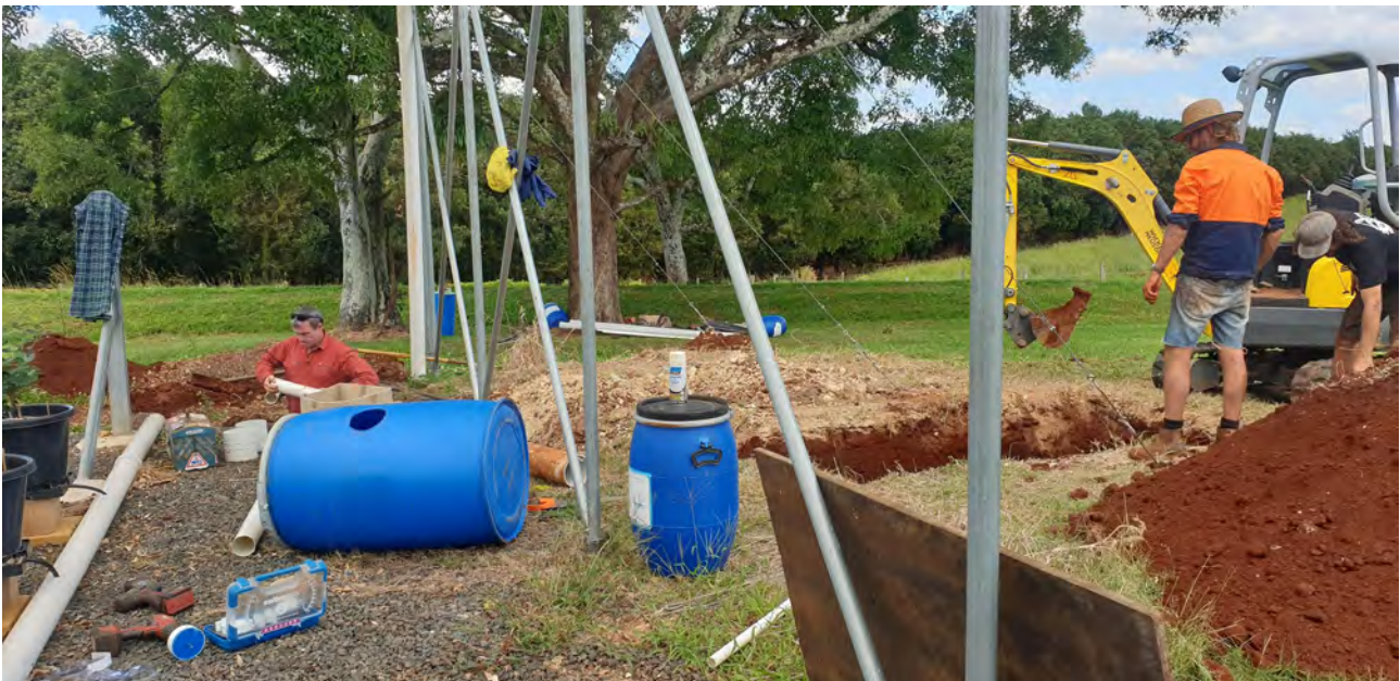
Installing pipes to drain waste water from 300 potted blueberries, into a sump tank that will feed the bioreactor and wetland structures, at the Wollongbar Primary Industries Institute. Photo credit: Diana Unsworth
